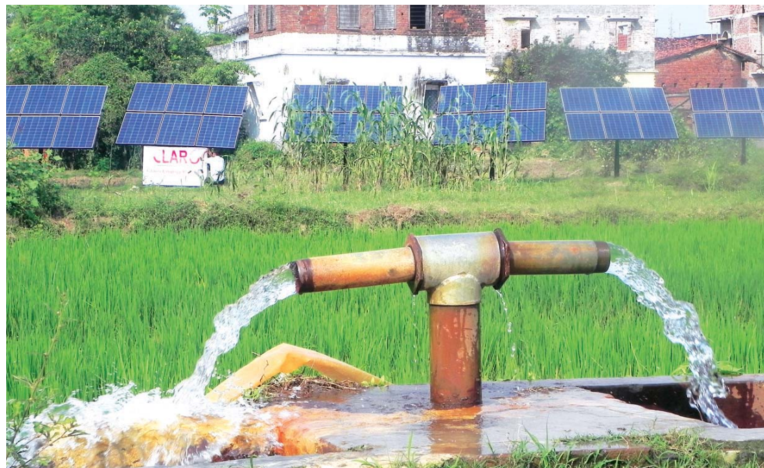
Solar-based pumping at work at a farm near Patna. Claro decided to target Bihar as it had high power deficits and being in the Gangetic plains, the water table was high — five metres after monsoon, and 10 metres in other months
